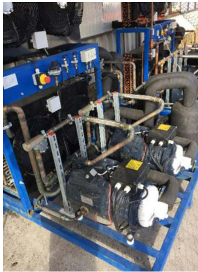
Fig.2: Compressor / condenser racks
