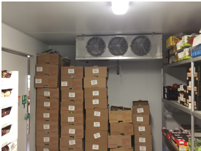
Fig.3: Evaporators / inside cold storage
